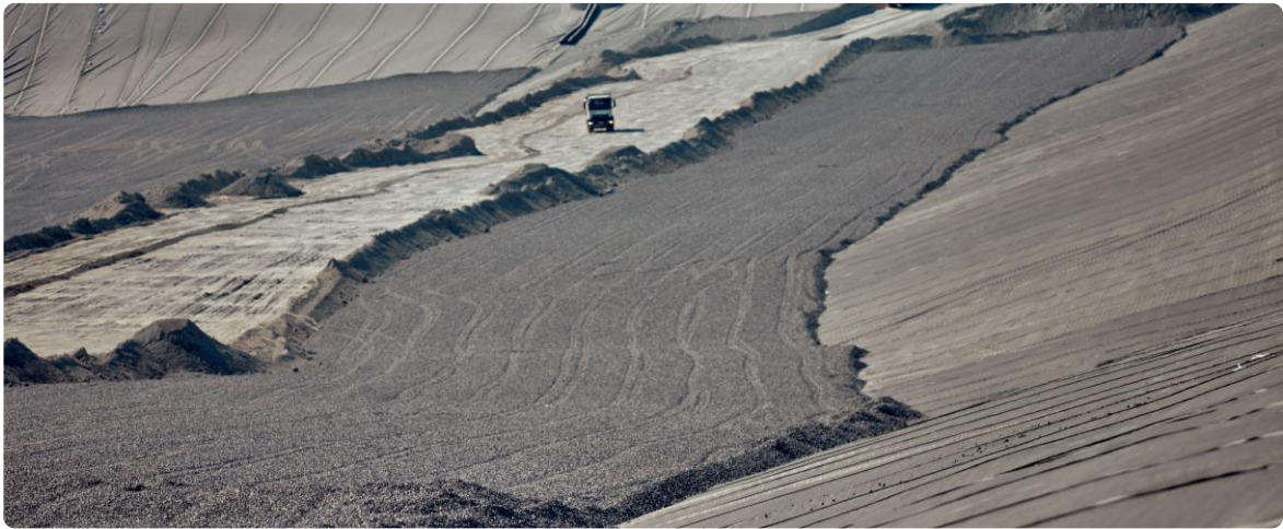
Sub-cell collection system
