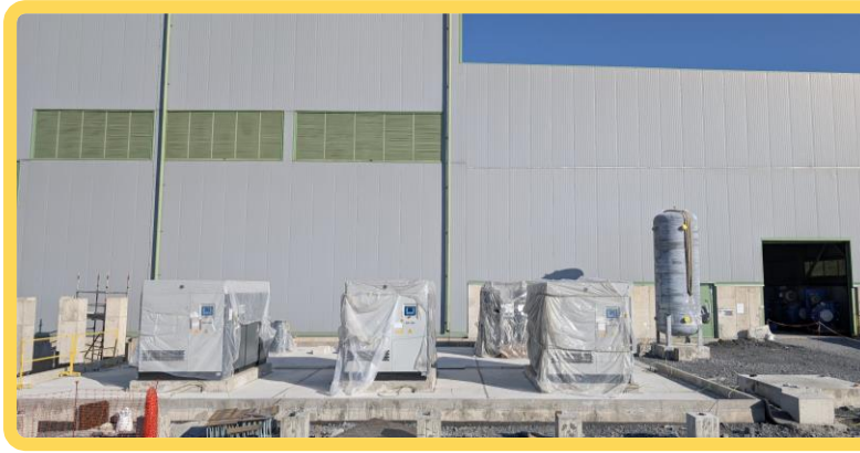
Process compressor building
